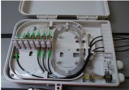
One of 6 connection boxes in a series configuration
